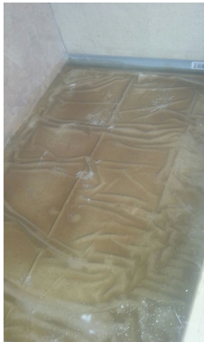
Figure 34: Wrinkles occurred when the molded part was left in the garage.
