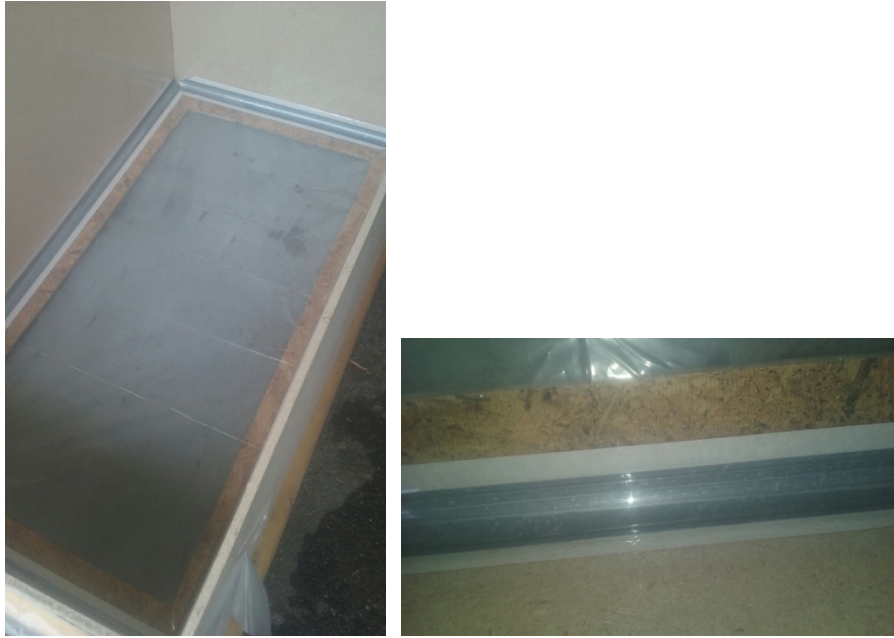
Figures 31: Round corner molds that are typically used in drywall applications, and we used it and taped it in the corners to have a molding part with no sharp edges.
